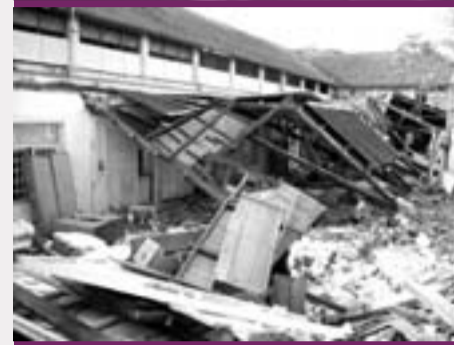
The annex to the old Dutch Hospital at the Old Town of Galle World Heritage site was destroyed by the tsunami
