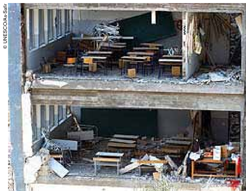
Damaged school in Bing Jbeil.
