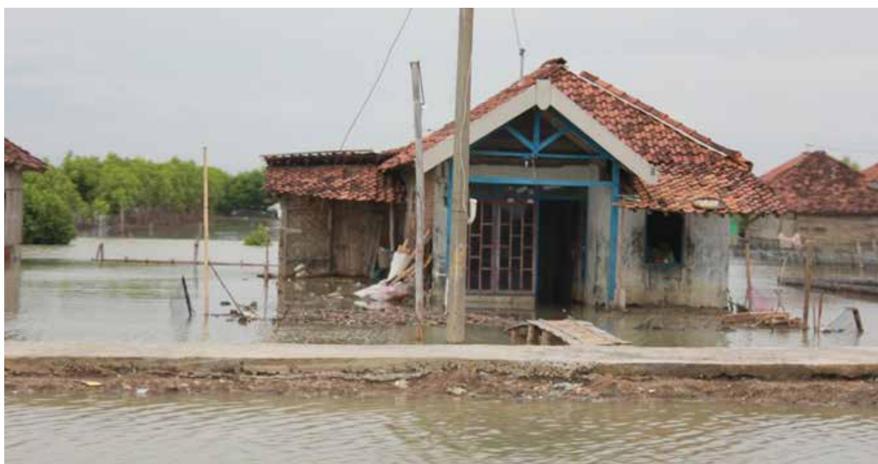
Figure 2.2.1: Coastal flooding in Bedono Village, Sayung, Central Java
