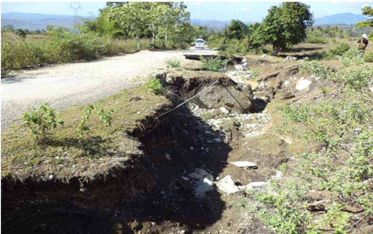
Figure 2.3.1: Roads damaged by frequent floods in Viqueque, Timor-Leste
