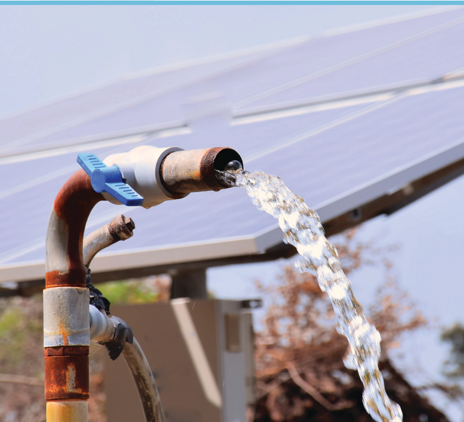
Equipment for a solar-based irrigation project.
