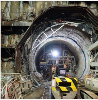
Engineering infrastructure, such as this underground metro tunnel, is essential for sustainable development. © Mr Pung Chun Nok, Hong Kong Institution of Engineers
