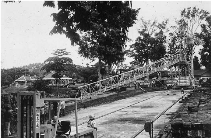
Photo 6.2.1.1 Rail track of the tower crane
